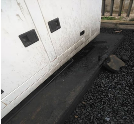
Figure 4a: Used engine oil spillage beside the generator.
