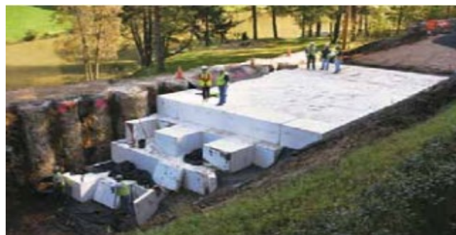
Figure 1: EPS applied to reduce stress and settlement on underlying subgrades (Aaboe and Frydenlund, 2011)
