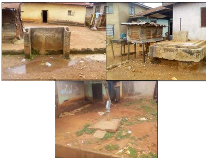
Figure 3. Damaged stand pipes and boreholes in Ado-Ekiti
